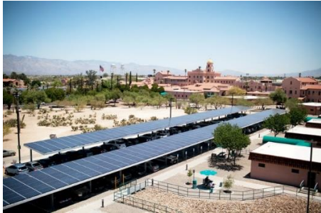
REC solar panels powering Tucson's veteran's hospital in Arizona, U.S.
