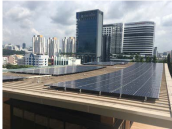
REC Group's solar PV system at the SSA roof.
